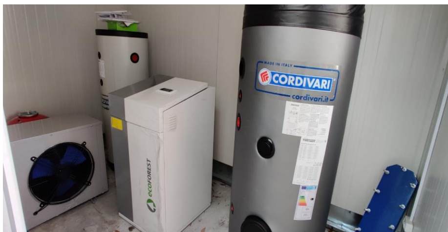
Figure 10. Preliminary positioning of the equipment in the container (technical room located close to the existing building)
