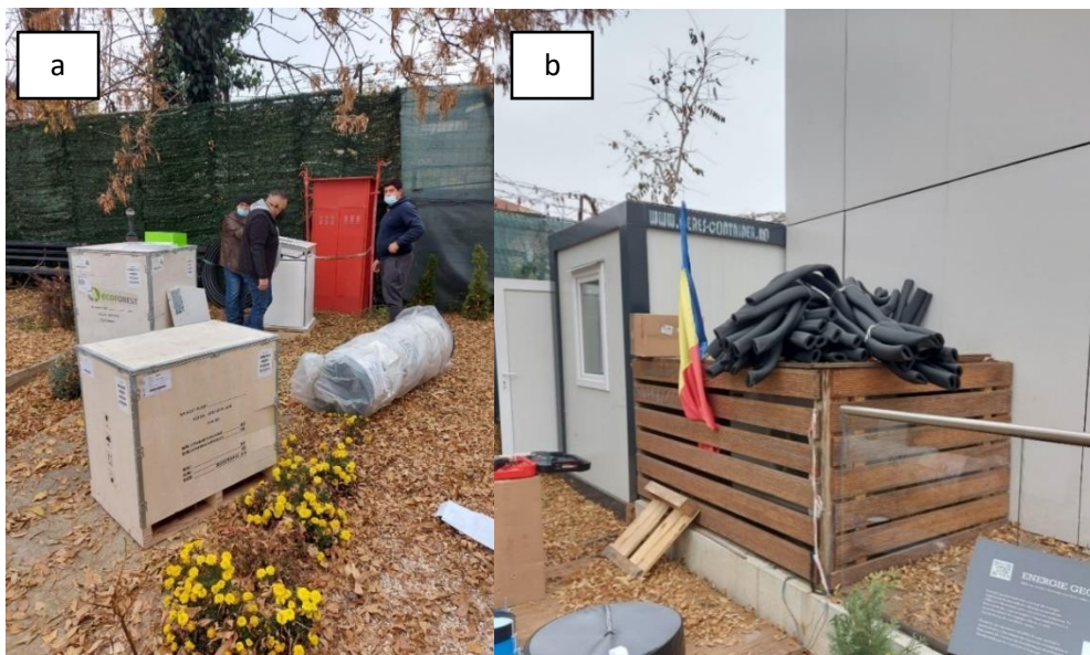
Figure 9. Unloading the pieces of equipment for the technical room (a) and the final positioning of the container on the concrete foundation slab (b)
